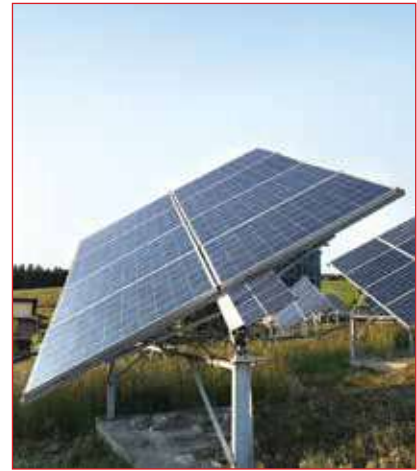
Solar PV System
